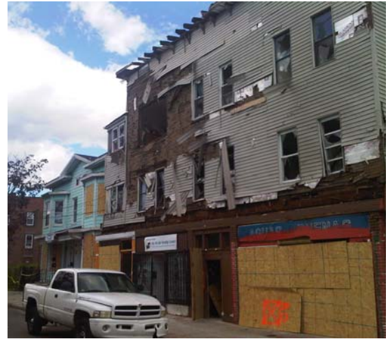
Damages to businesses and homes on East Main Street in Bridgeport, CT caused by the tornado.
